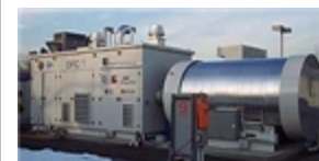
FuelCell Energy Sells Megawatt Power Plant to Turlock Irrigation District in California
